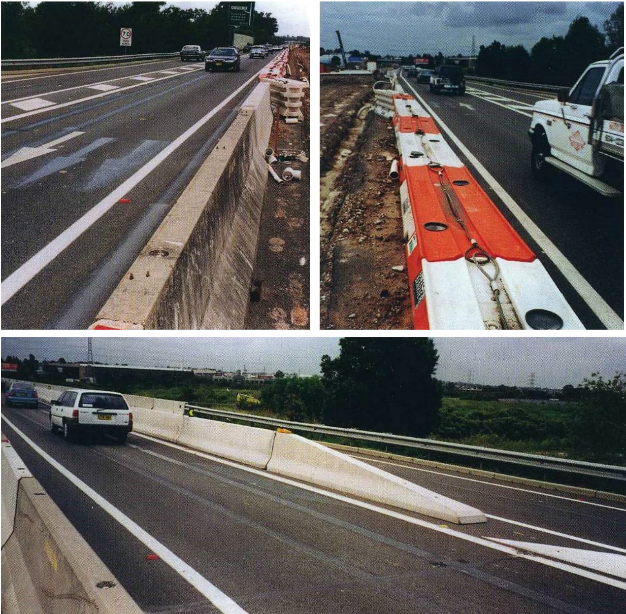
Figure 3.4: Example barrier type and installation identified by road safety audit as unsafe
